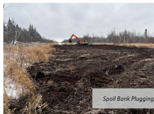
Woody Debris Plugging
