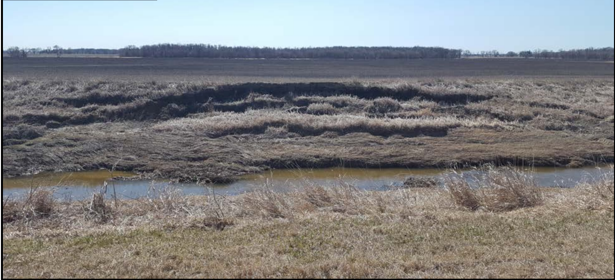
Example of Failing Ditch Banks along Polk County Ditch 2
