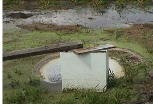
36-4B Water Control Structure
