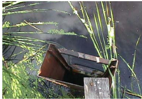
4-6B Water Control Structure
